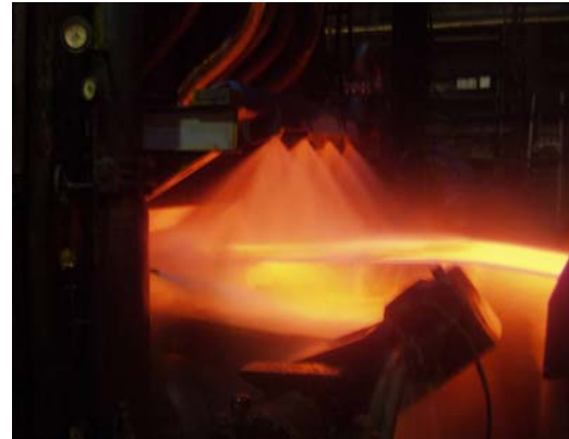
Figure 2. Interstand cooling header with full cone nozzles
