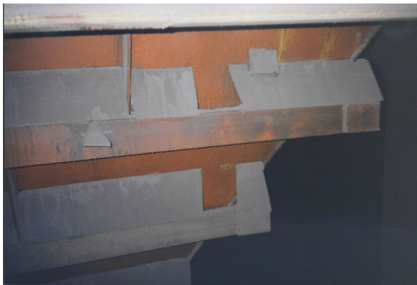
Figure 8. Corrosion damage of hopper walls
