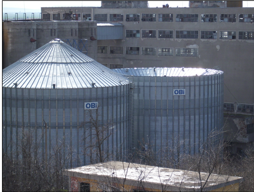
Figure 7. Bend of the silo roof
