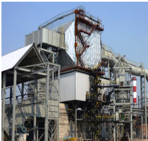
Figure 3. Electrofilters of dust exhausting plant of BF-8
