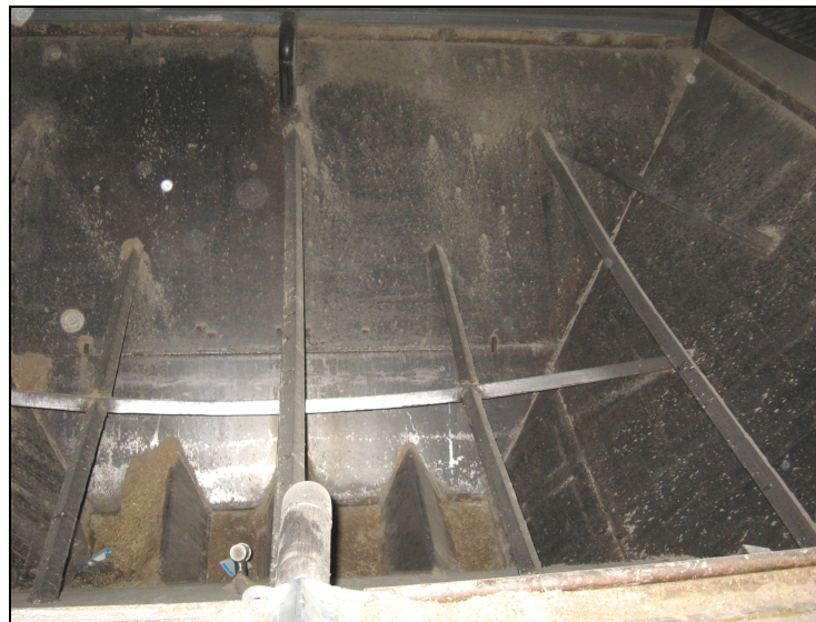
Figure 4. Deflections of the retaining steel strands of unloading hoppers of the capacitive structure
