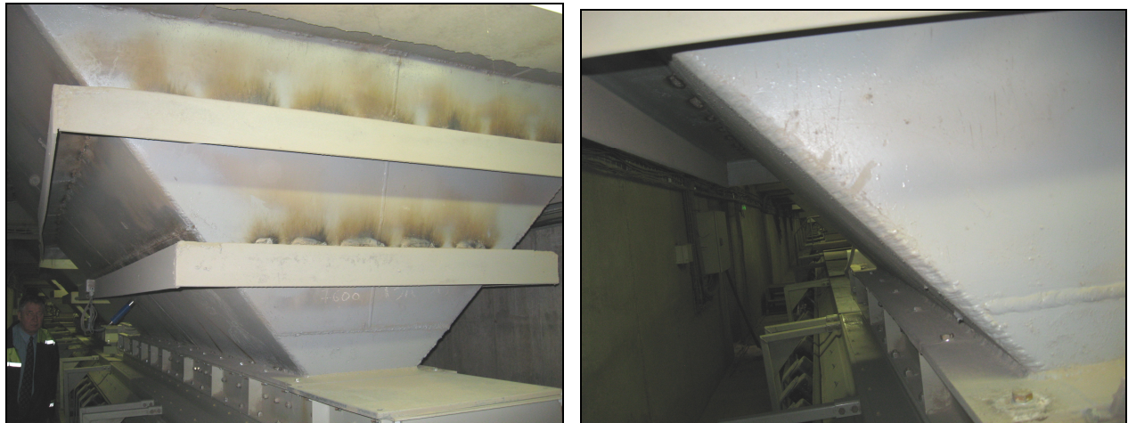
Figure 3. Deflections of the bearing elements of unloading hoppers of the capacitive structure
